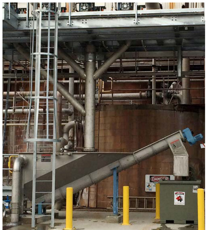
The SansGrit operating in a mill
